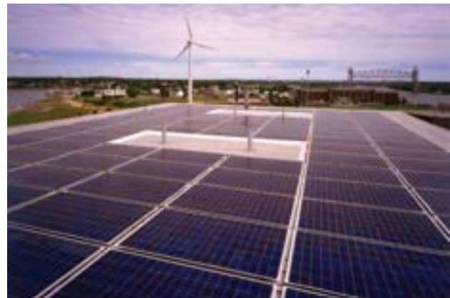
Rooftop Solar Array, Company #1 and #2 at Mass Maritime
